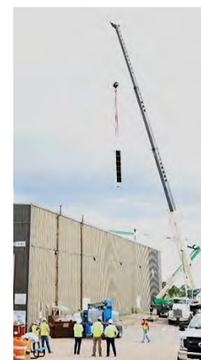
Figure 2.2.7.2.2: The cleaning of the 4 motor generator coolers required removing each 16-foot tall and 7,500lbs. cooling towers via a small hatch in the roof above each corner of the motor generator. The teams responsible for this high consequence operation included LANL, PFF, and external contactor personnel.
