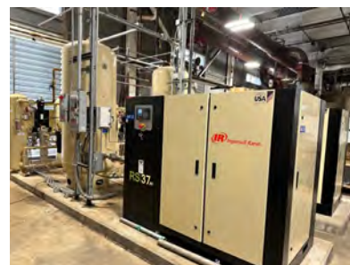
Figure 2.2.2.2. Air compressors, receiver tanks, and dryers are located in the DCFF plant.
