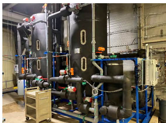
Figure 2.2.2.1: New magnet cooling water treatment system
