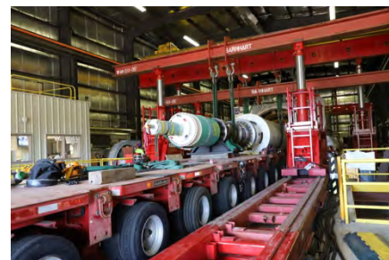
Figure 2.2.7.1: The removal of the 1.4GW motor-generator rotor in preparation for a full inspection at GE in Richmond, VA.
