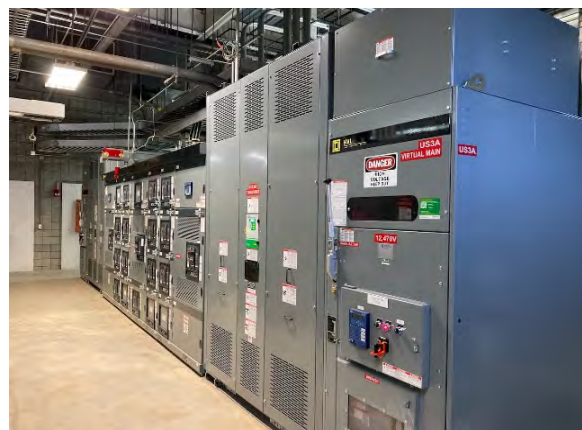
Figure 2.2.2.2: Three-phase 12.5kV-480V switchgear
