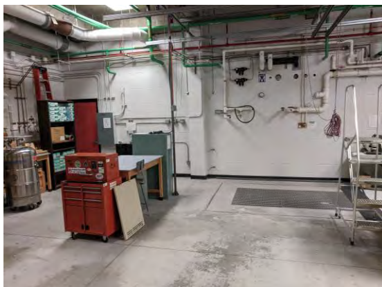
Figure 2.19: An August 2020 view of the future location of the Fast-Turnaround Facility in NPB B135. A 10ft deep, 3ft wide floor pit is visible.
